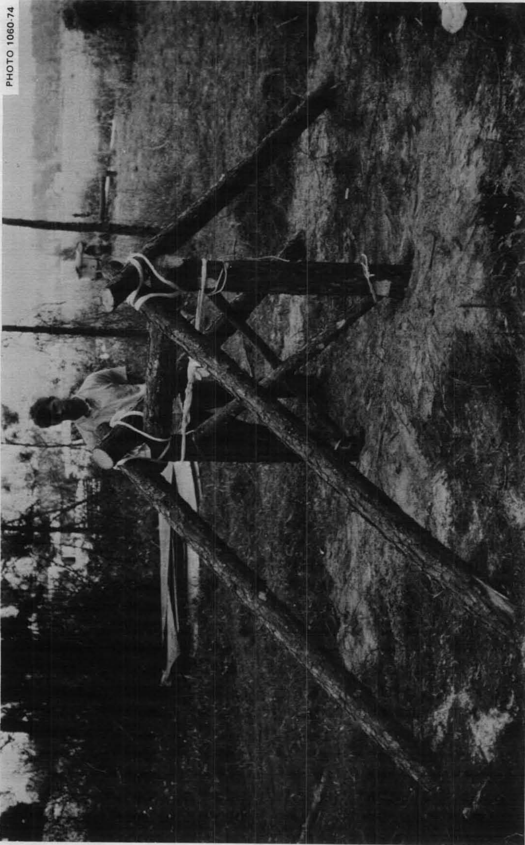
Fig 5.31. A second prototype of the frame of a Ridge-Pole Shelter, built without using a single nail. Slightly twisted strips of bed sheet, 1 ft wide, were used to hold this simple yet very stable structure together, and three pieces of rope were used to secure the notched cross-braces between the two vertical posts supporting the ridge pole. These vertical posts rested on flattened small areas cut on the upper side of a slightly below-ground footing log. Small poles on the outer side of the vertical posts, just below ground level, prevented any sideward movement of the bottoms of the vertical posts.
